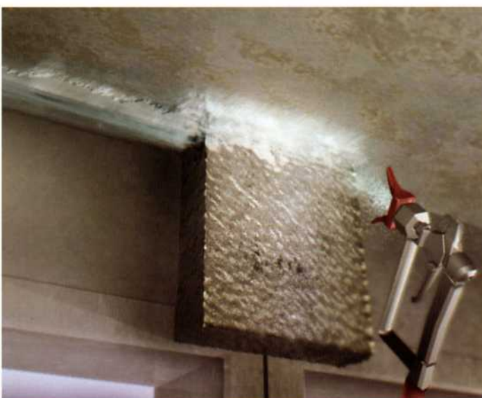
SpecSeal® AS205's unique viscosity characteristics allowed it to be applied to the underside of the safing and floor with minimal dripping.
